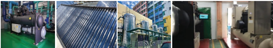
Green Chiller , Hospital Setiu
